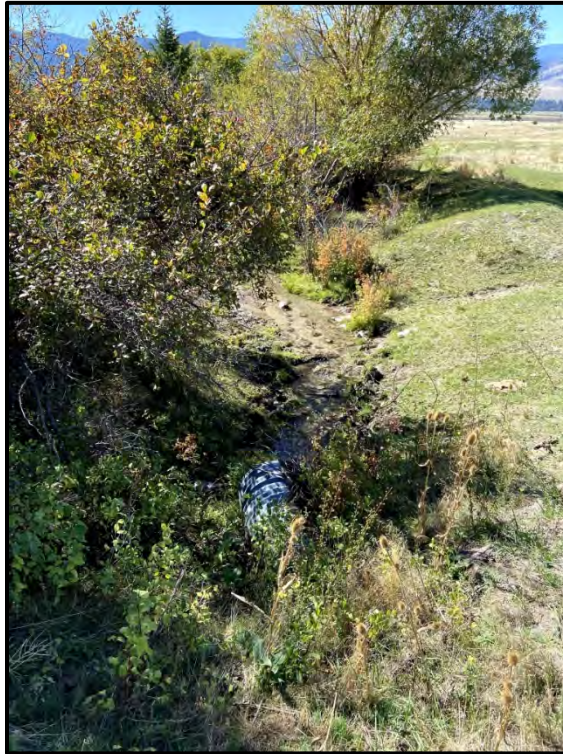
Photo 11: View of Lamoose Creek (TRIB 1) where it is routed under the K Canal and outlet through a culvert to the south.
